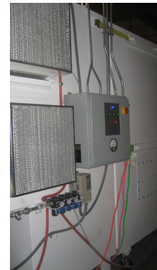
RPC Collector Showing Final Filters and Control
