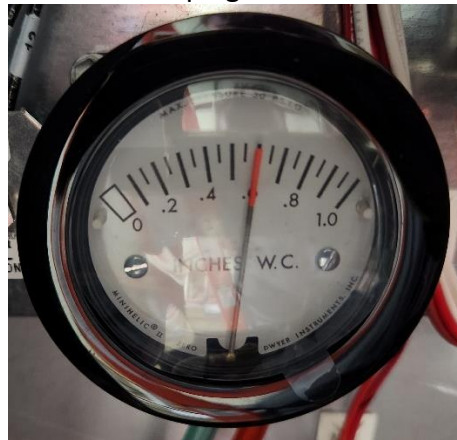
Manometer reading .6" w.c. air pressure across the burner profile opening.
